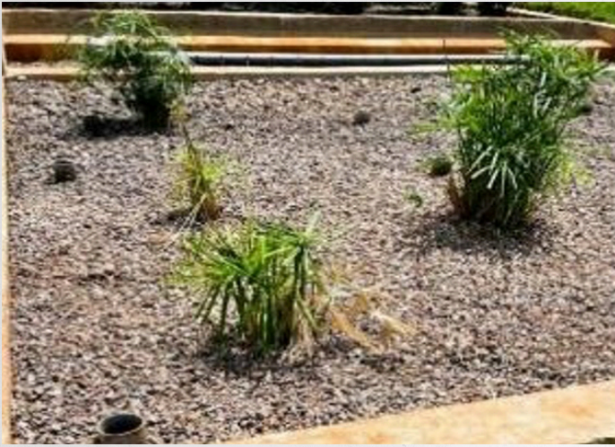
Wetland treatment starts with a holding tank, then a vertical flow bed and a horizontal gravel bed.
