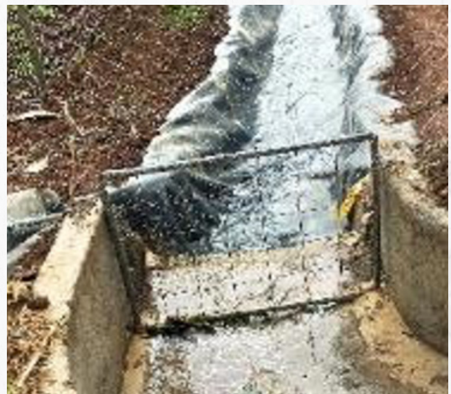
Stormwater and irrigation run-off to the wetland treatment system by way of lined canals.
